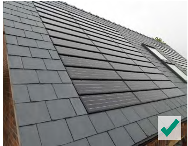
Figure 48: Integrated solar panels on slate roof.
