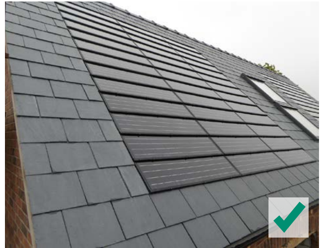
Figure 48: Integrated solar panels on slate roof.
